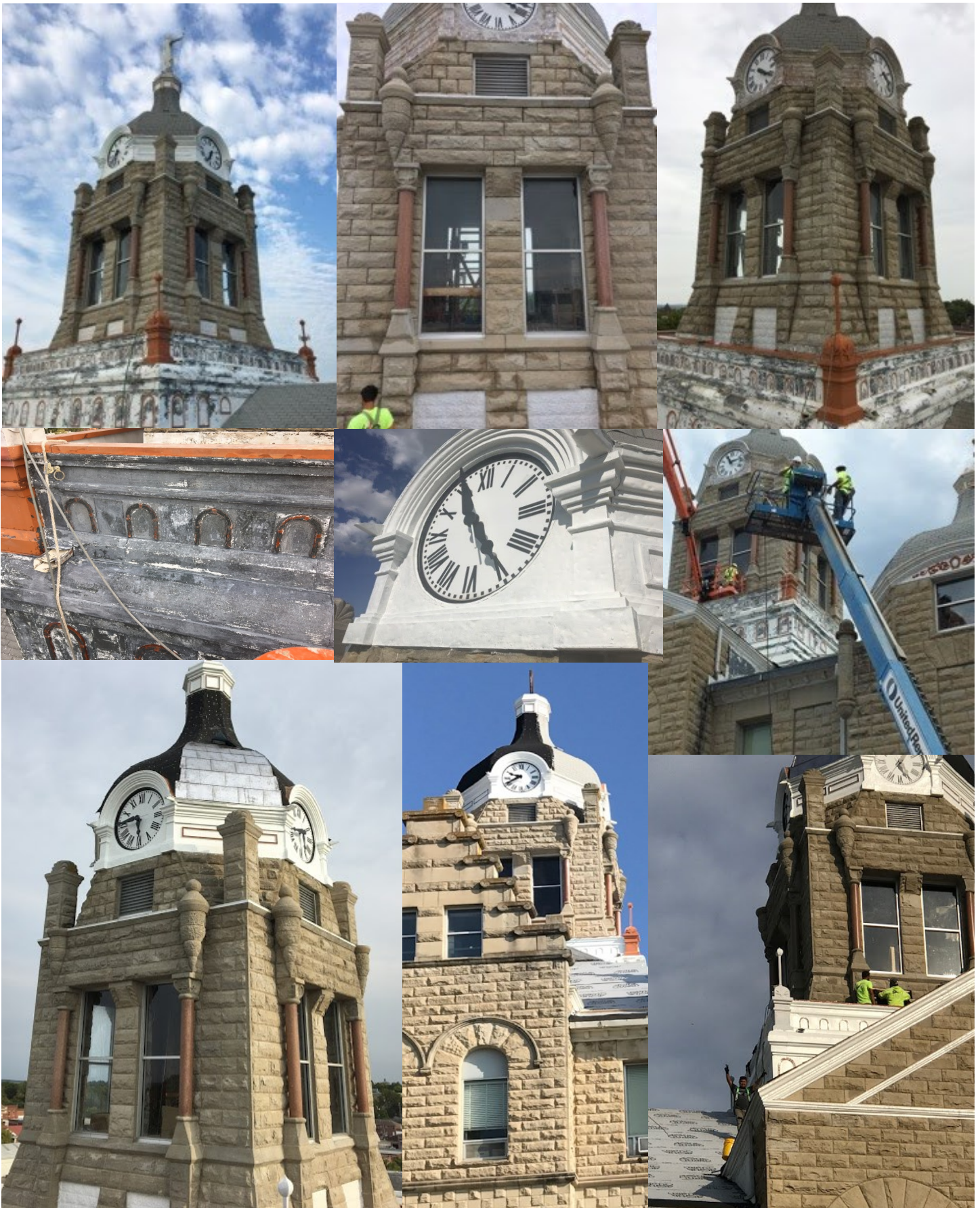
Tower: Clocks being primed and painted. Partial roof torn off and papered in. Four sides of lead coated copper flat lock pans started.
